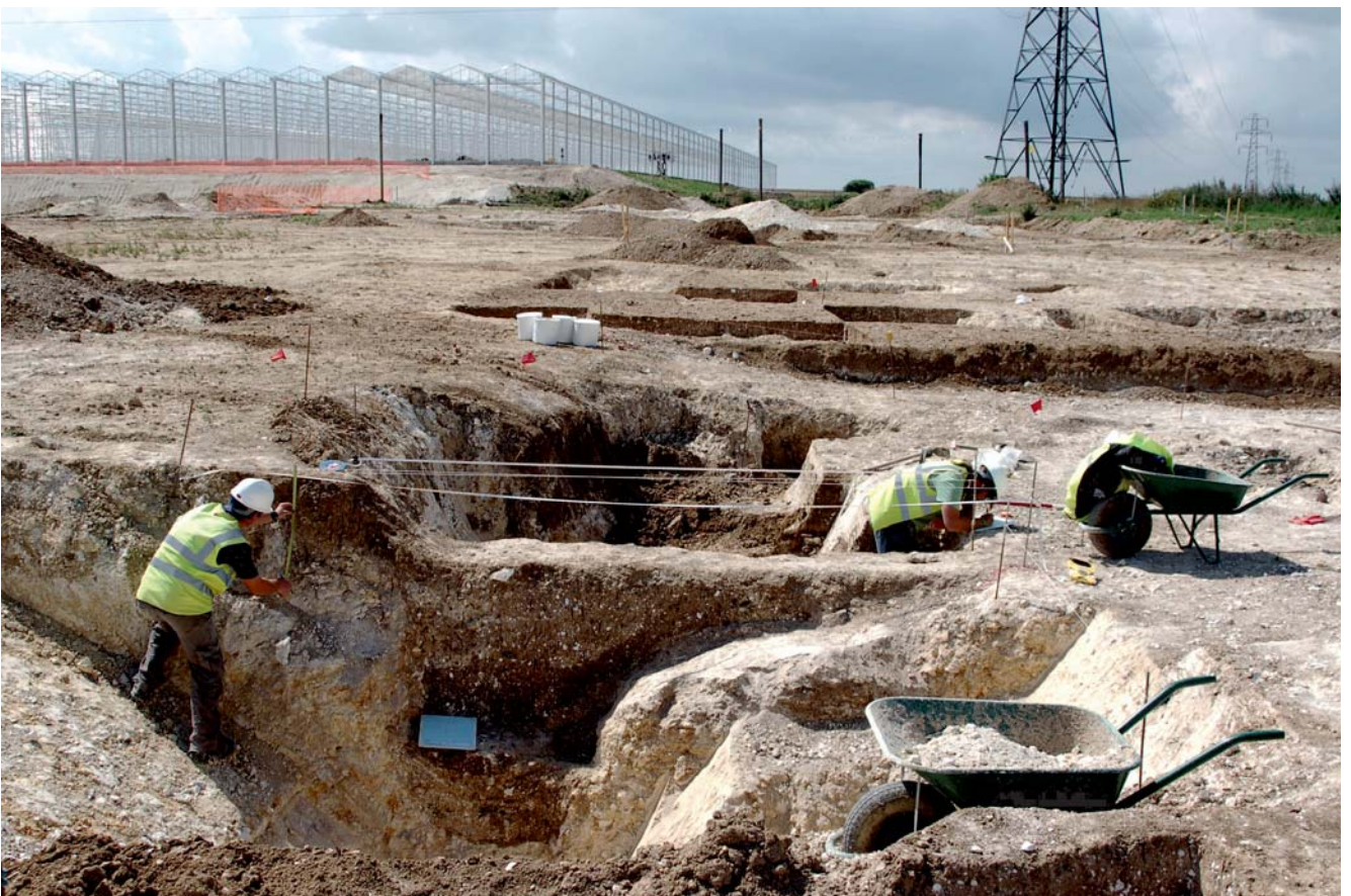
Plate 252. Site 7, excavation of the underground chambers (G1221, G1219 & G1228) & other features, looking south.
