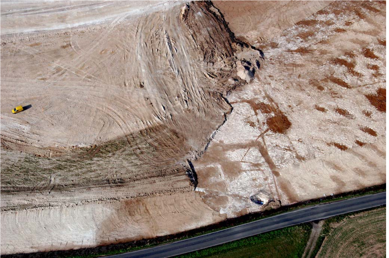
Plate 309. Site 17. Aerial view after the topsoil strip showing most features including a water main trench, looking north-west.
