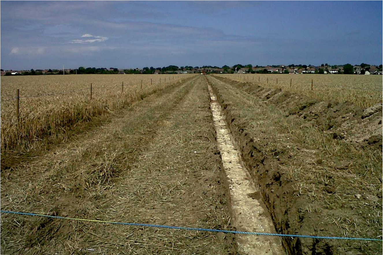
Plate 15. The plateau south of Birchington traversed by the pipeline trench. Looking north-east towards Birchington.
