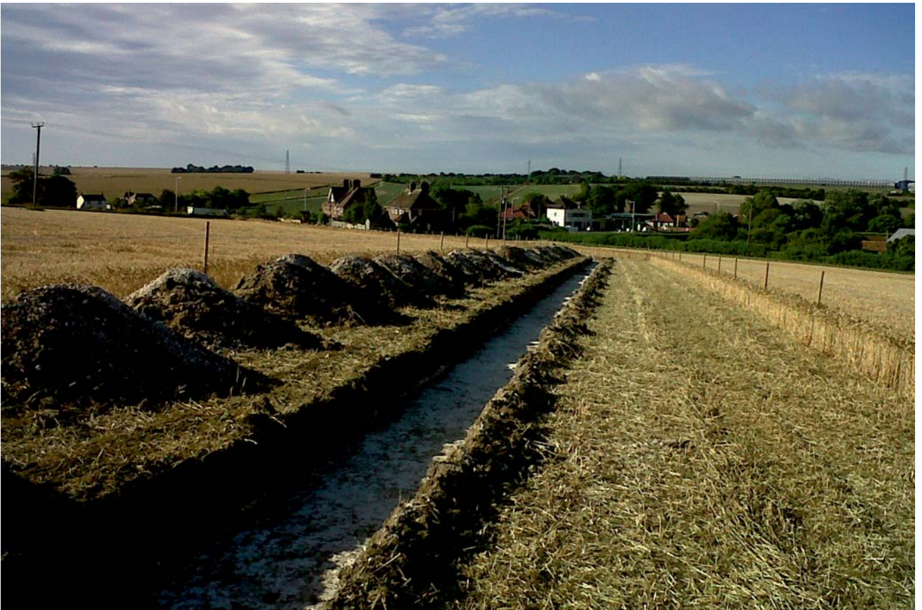
Plate 14. Downland landscape traversed by the pipeline trench. North of Little Brooksend, looking south towards Thanet Earth.
