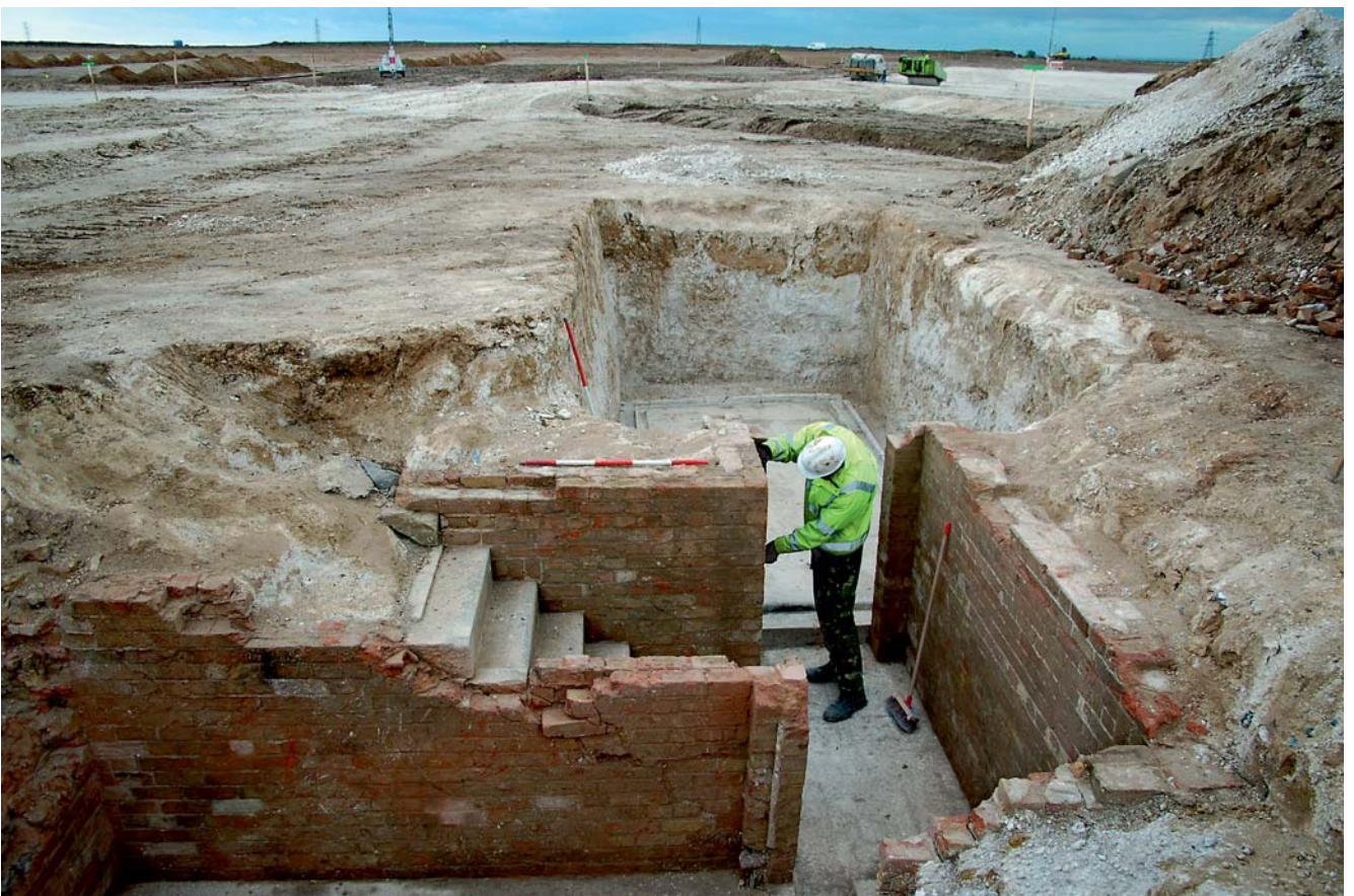
Plate 344. Second World War Structure 61 (G4096). Detail of Room 1 & access steps, looking south (scales 1m & 2m).
